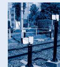
踏切障害物検知装置 Crossing Obstructing Detector
